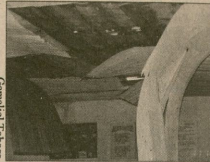
The ceiling of this CLEAPS classroom was not spared by typhoon Katring
